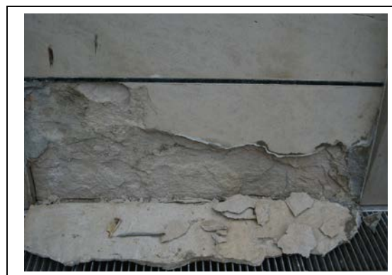
Structural Damage at Creekside
