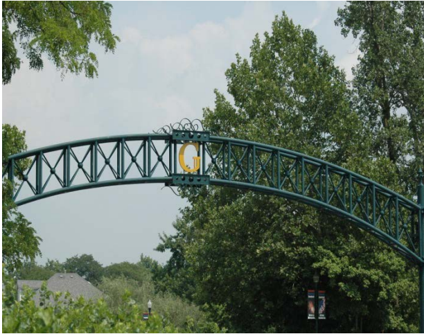
Gateway Arch over 62
