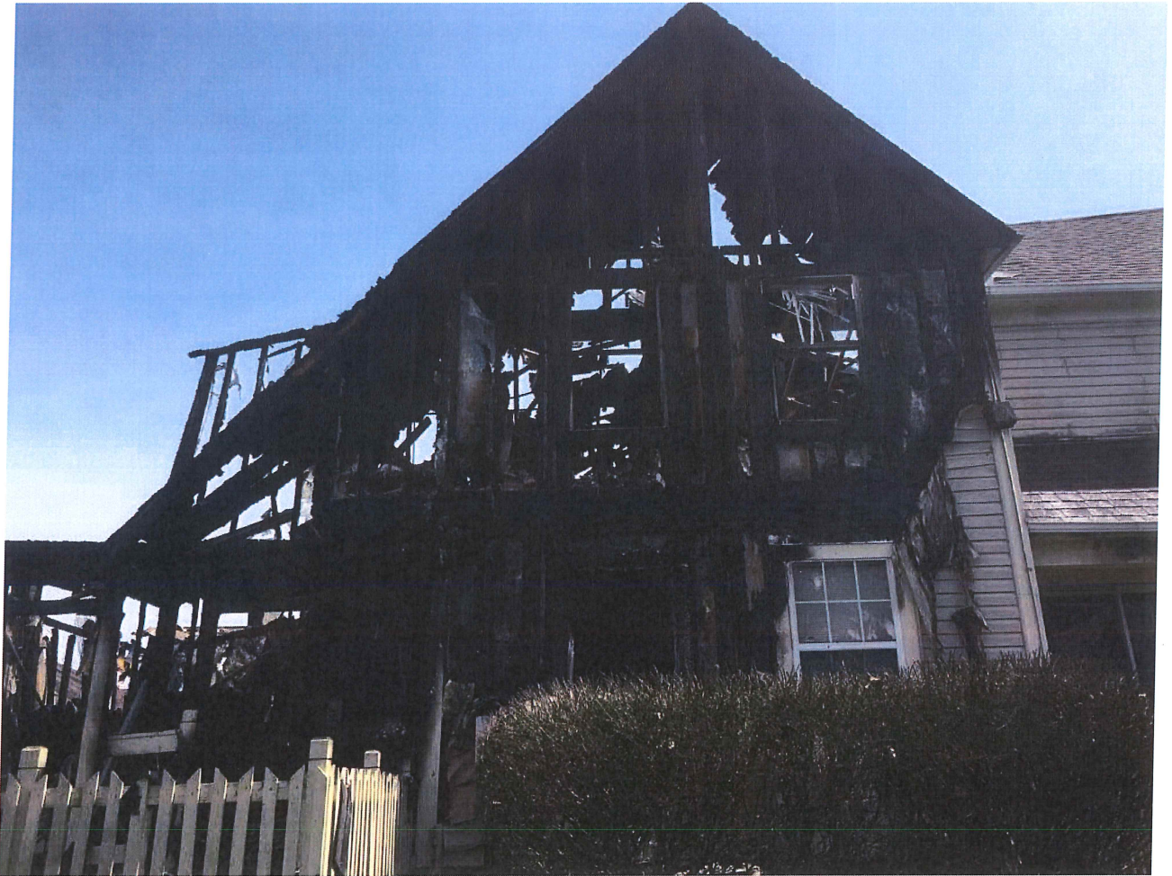
Second Alarm Fire – 303 Vista Drive. Saturday April 21, 2018, 0105 hours.
